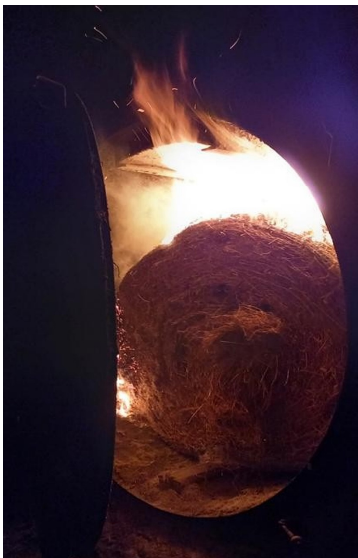
Combustion of large round bales of RCG in a batch fired biomass boiler
