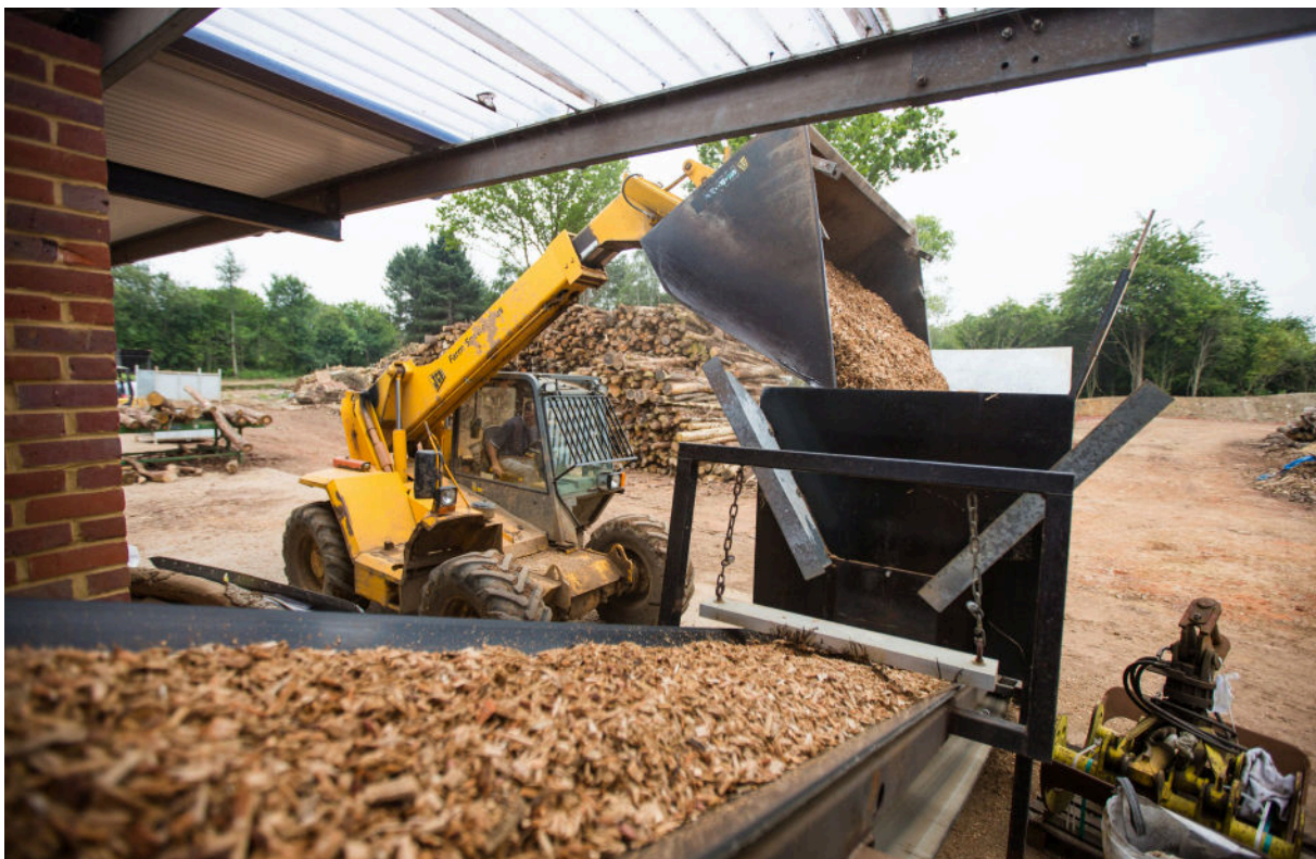
Figure 2: Chipped wood used to feed biomass boilers being fed into the hopper
